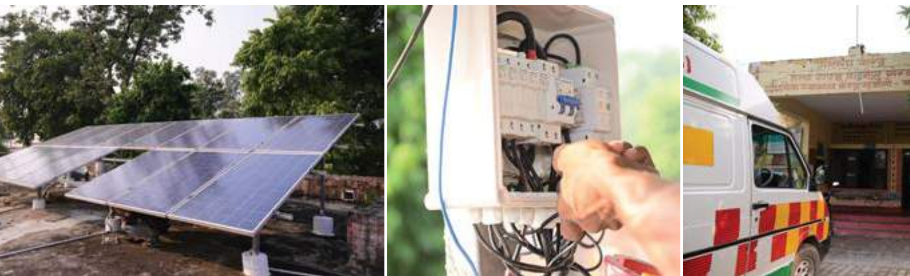
Brother's Brother Foundation funded the solar panel installation on a Primary Health Clinic in the village of Sujauli, Uttar Pradesh, India, to provide reliable access to energy.
